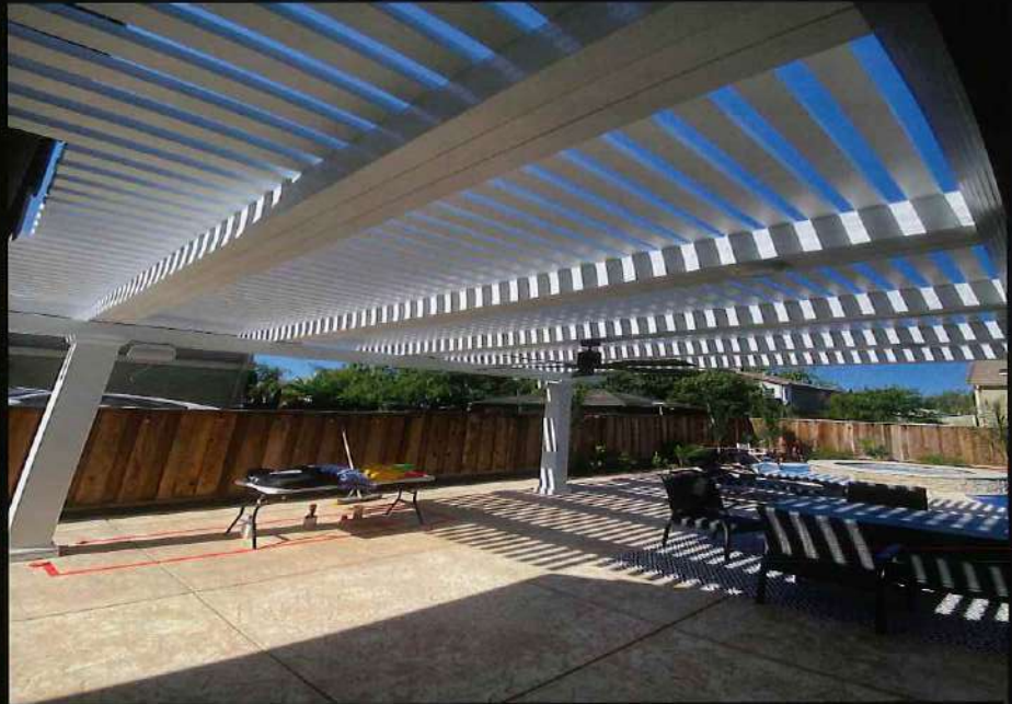
Ultra Lattice cover with 3x3 tubes, 3x8 triple rafters, 10" square columns, and double 3x8 beams.
